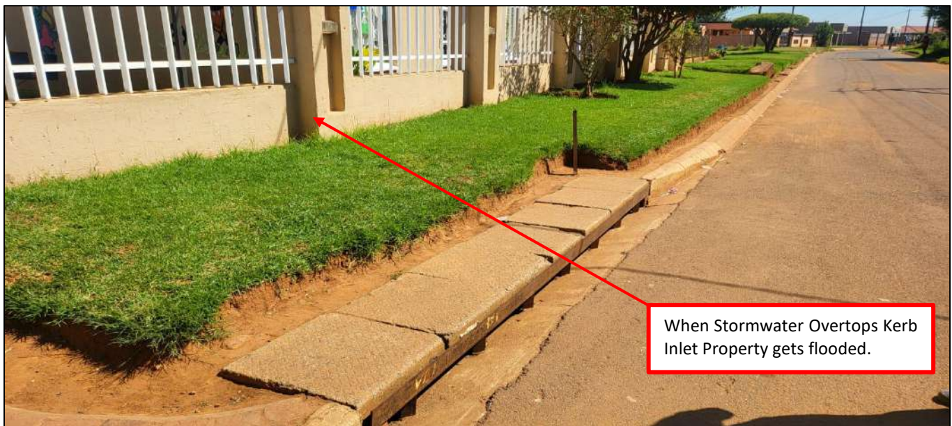
Figure 22: Low Point Kerb Inlet with Insufficient Capacity to Drain
