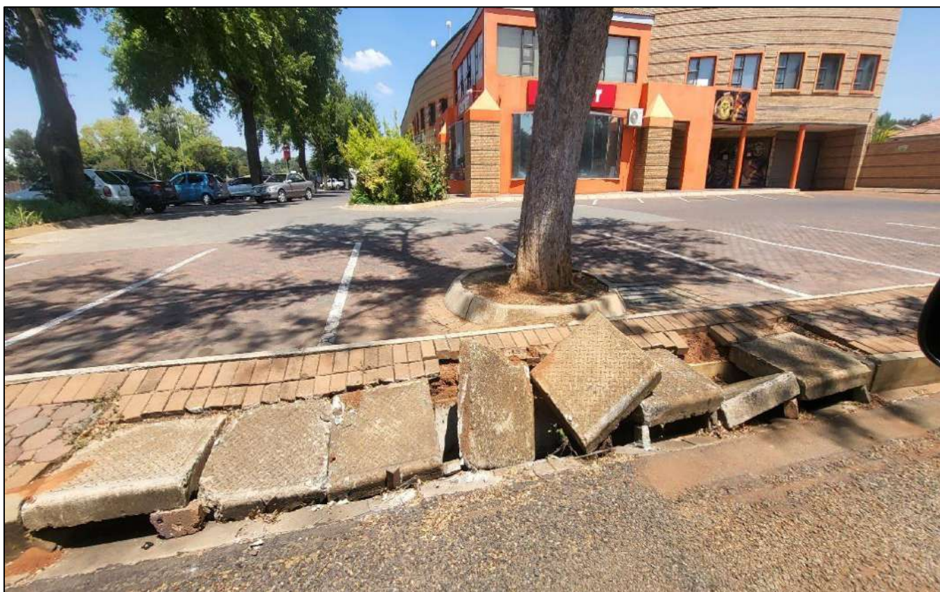
Figure 12 : Lack of Kerb inlet repair leading to stormwater not effectively conveyed from road surface.
