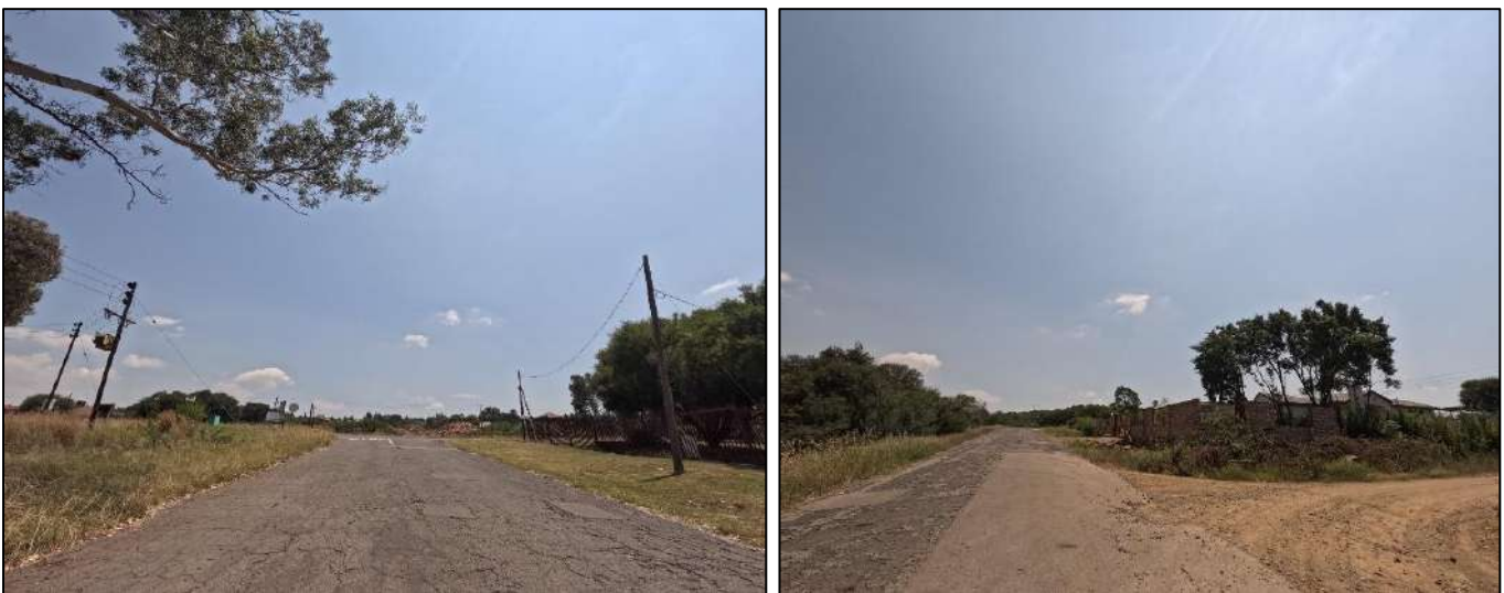
Figure 40: Lack of Stormwater and Ageing Asphalt Surface Leading to Edge Breaks.
