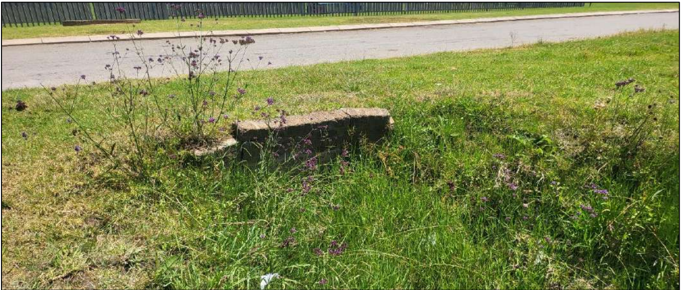
Figure 13 : Unlined SW Channel not maintained regularly Blocking Stormwater flow.
