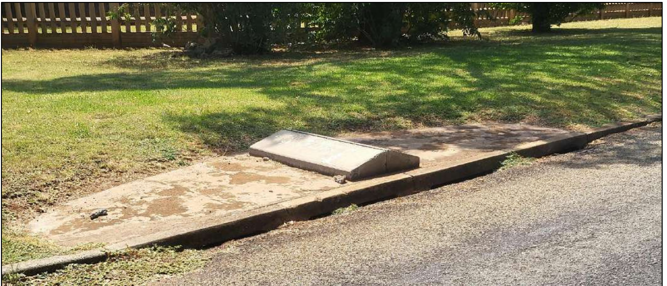
Figure 14 : Kerb inlet not raised when asphalt overlaying was done in the past.
