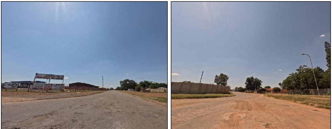
Figure 37: Surface Road Deteriorating and Washing Away of Surface Road
