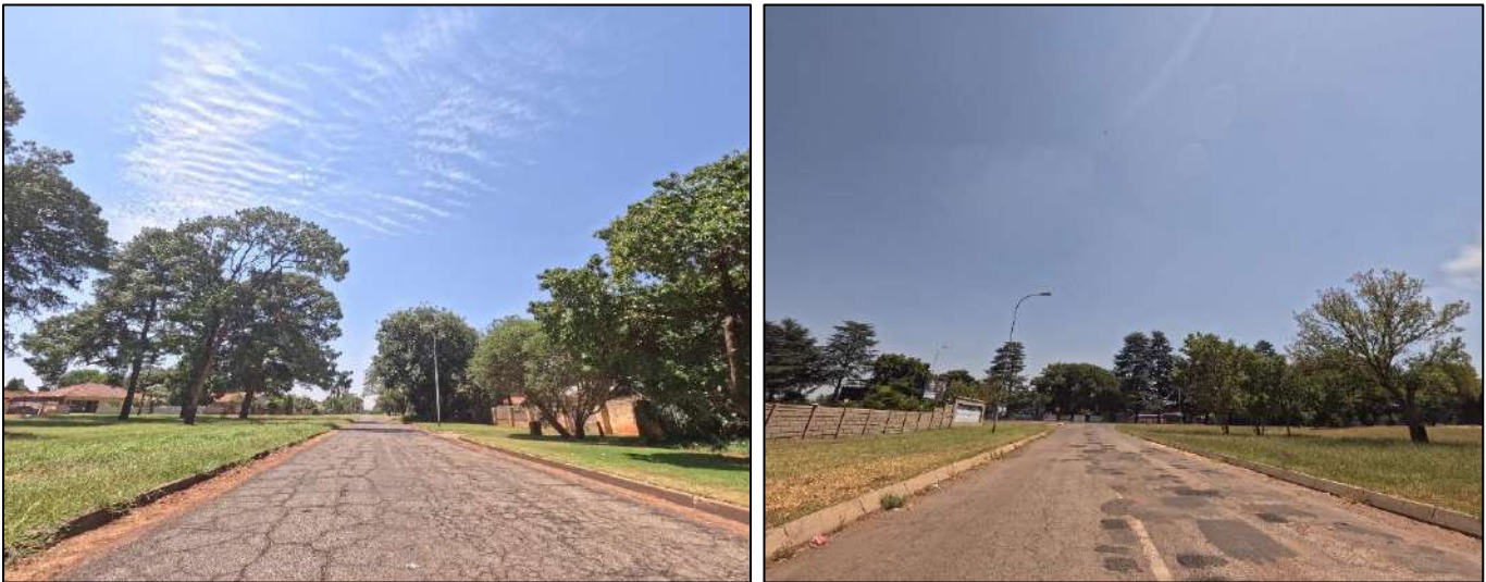
Figure 44: Damaged Surfaced Roads and Continuous Patching
