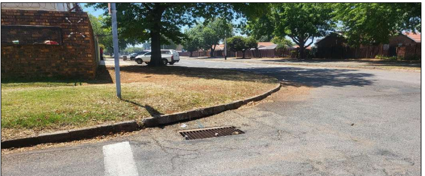
Figure 15 : Grid inlet in road surface of substandard size, prone to blocking by small debris.
