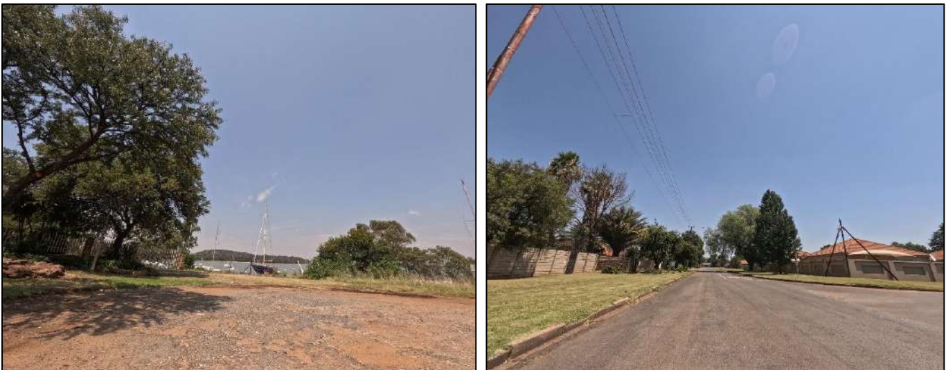
Figure 45: Road Deteriorating and Broken Kerbs
