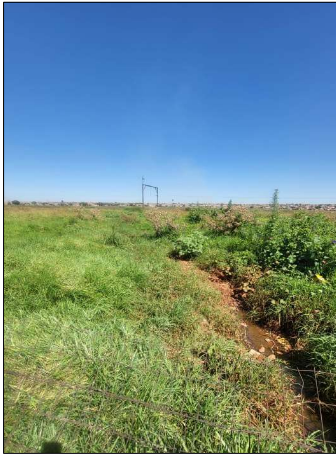
Figure 27: Down Stream Stormwater Discharge Channel Blocked
