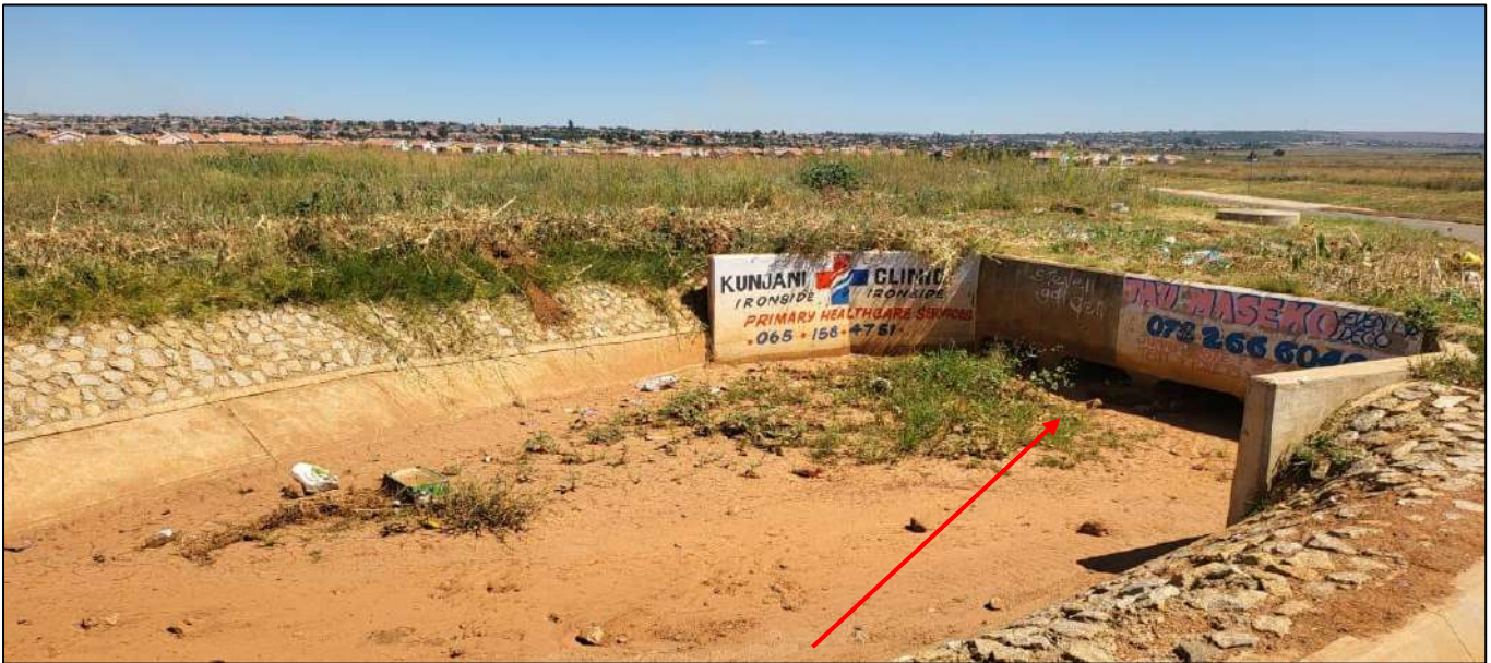
Figure 24: Stormwater Channel Culvert Blocked due to Lack of Maintenance
