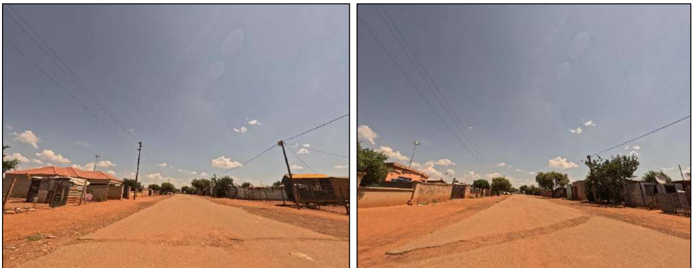
Figure 38: Road Crossings Not Properly Reinstated
