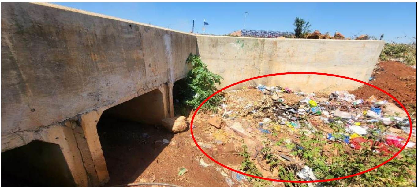
Figure 25: Stormwater Culverts Blocked due to Lack of Maintenance
