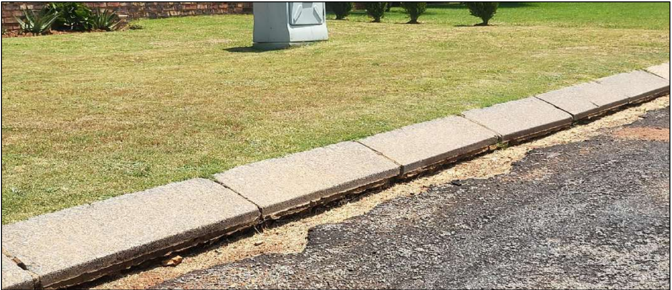
Figure 39 : Lack of Stormwater and Ageing Asphalt Surface Leading to Edge Breaks.
