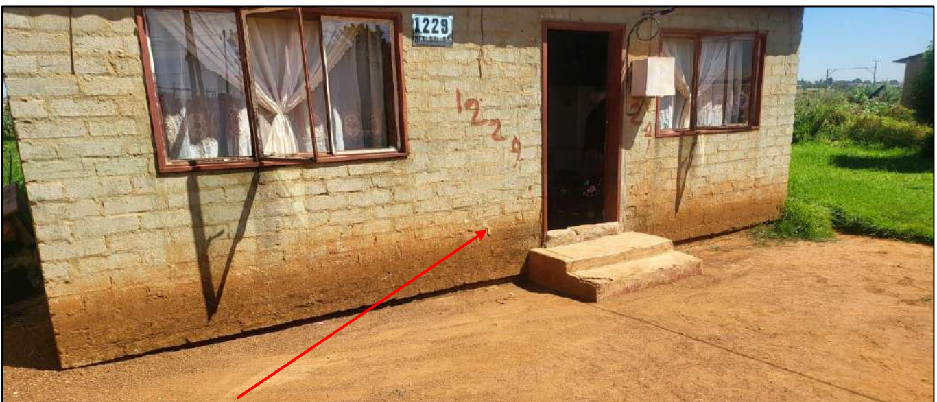
Figure 26: Stormwater flooding Level on Existing House
