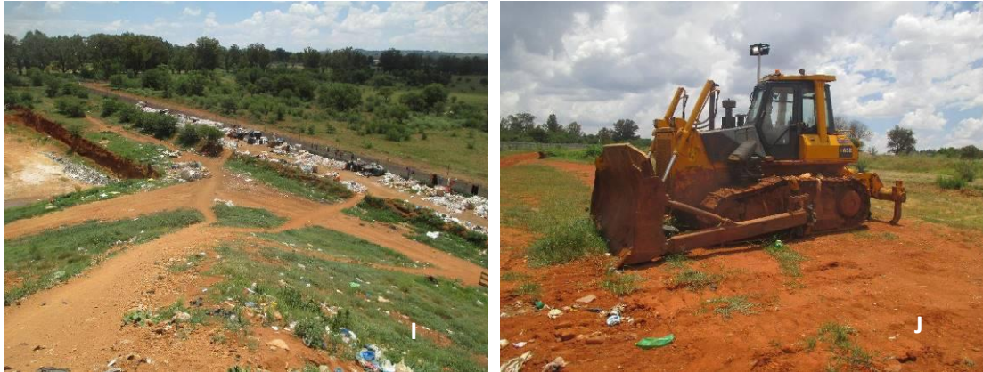
Figure 25: Photo A. Uncovered waste noted. Photo B: steep waste body. Photo C: incoming building rubble used as cover material. Photo D: incoming building rubble dumped in wet cell. Photo E: stormwater channel. Photo F: exposed waste at the edge of the waste body. Photo G: A prefabricated weighbridge kiosk on site. Photo H: informal recycling occurring on site. Photo I: scavenging occurring on site. Photo J: non-operational bulldozer on site.
